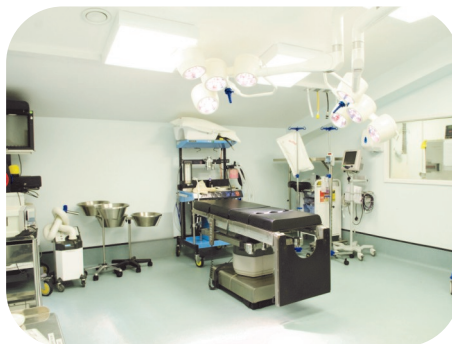
One of our purpose built operating theatres.
